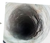
2 weeks after Vulcan was installed, scale had been softer and fallen out.
