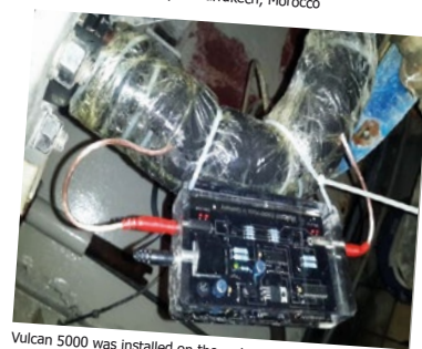
Vulcan 5000 was installed on the water inlet of the water recycling room.
