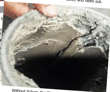
Without Vulcan, the filter was quickly stuck by scale deposits, and it had to be changed every 48 hours.
